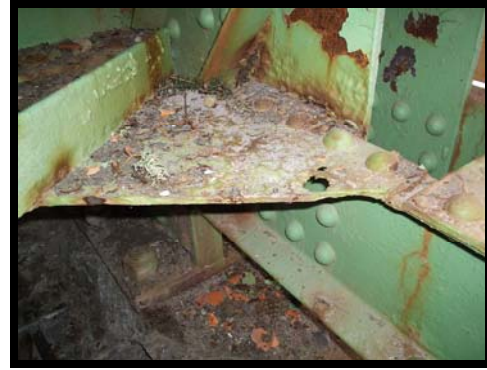
Corrosion of a structural connection
