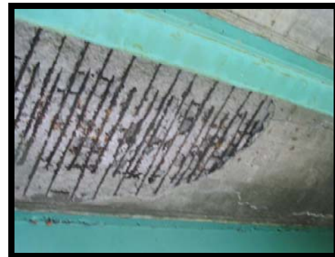
Concrete spalling and exposed reinforcing steel
