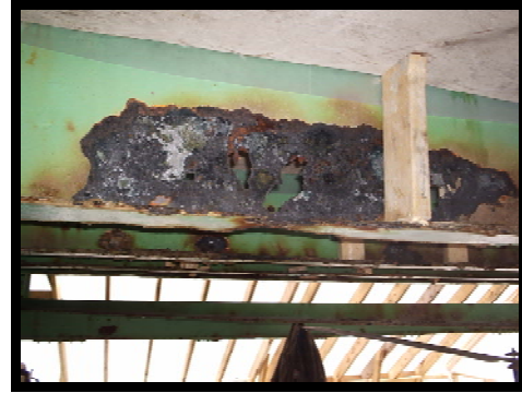
Advanced corrosion and section loss
