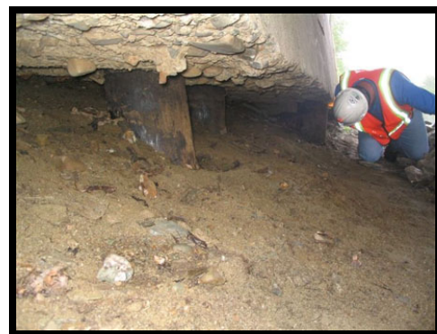
Abutment scour with exposed timber piles
